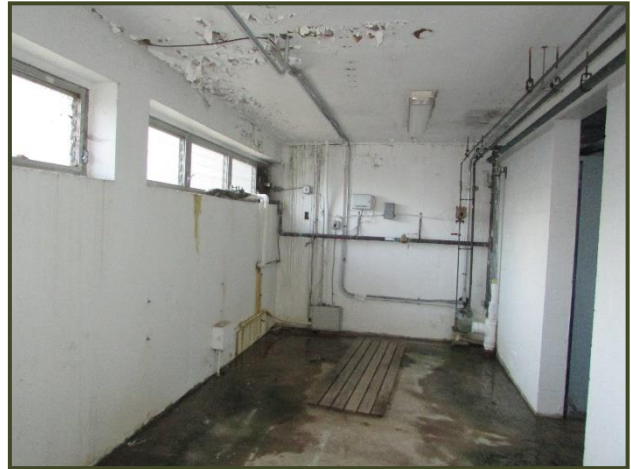
Photo No. 25 – Water infiltration in pool locker room
