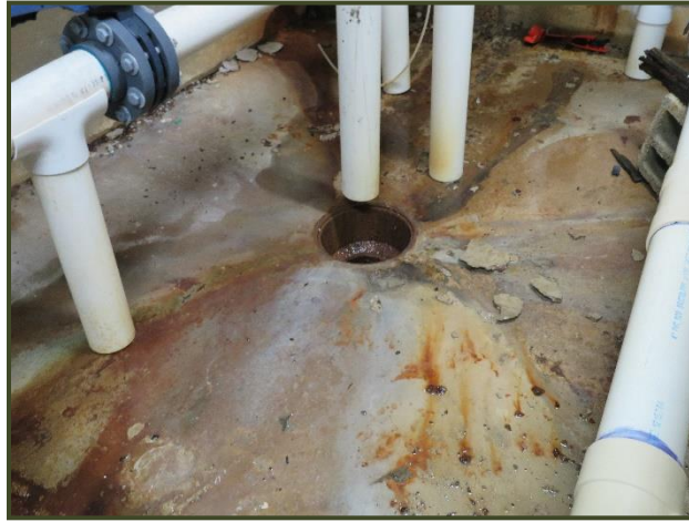
Photo No. 28 - Corrosion staining and efflorescence present at pool pump room drain
