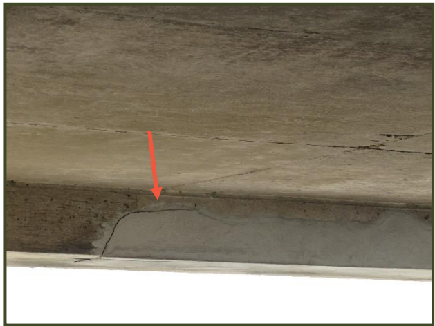
Photo No. 11 – Failing previous patches on concrete equipment pad
