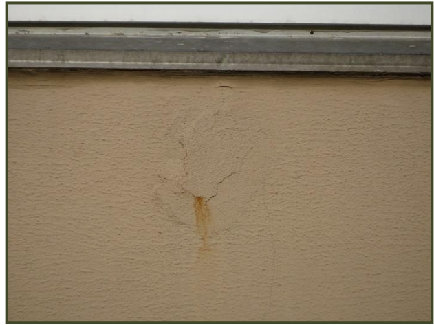
Photo No. 16 – Incipient spalling and corroding reinforcing at concrete framing
