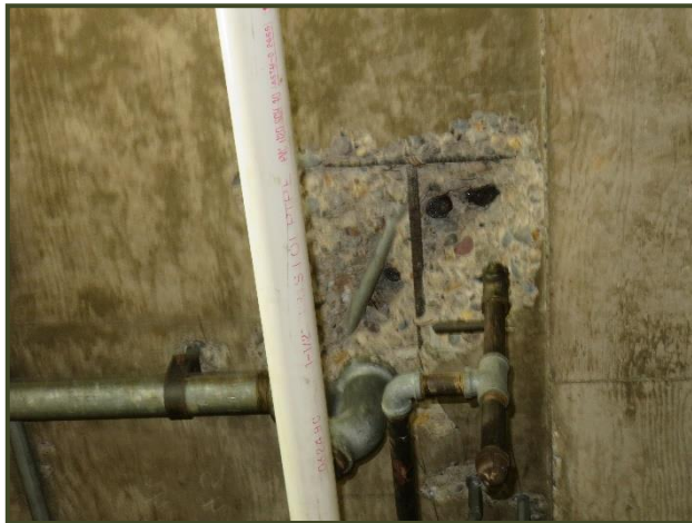
Photo No. 1 – Concrete spalling and exposed reinforcing at roof penetrations
