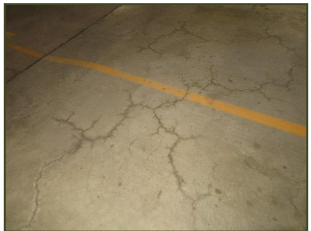
Photo No. 6 – Map cracking in concrete slab on grade
