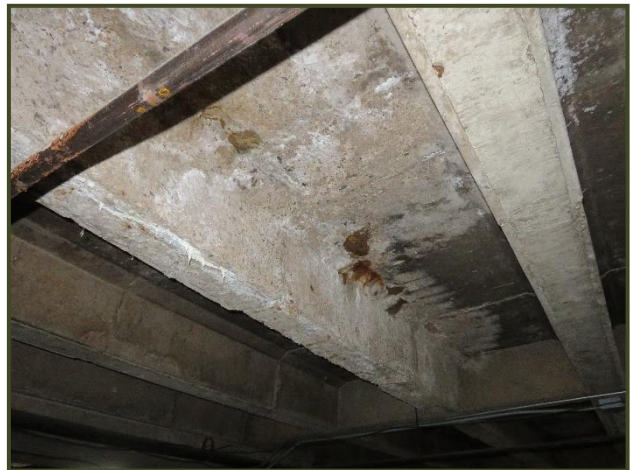
Photo No. 4 – Concrete spalling and water staining at parking garage ceiling
