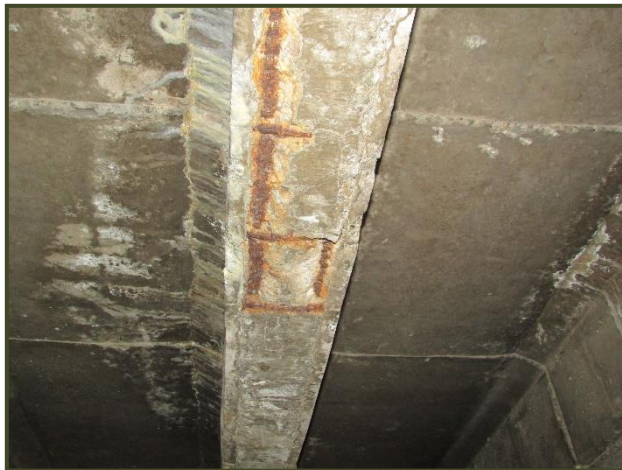
Photo No. 3 – Concrete spalling and exposed reinforcing in concrete beam; water staining
