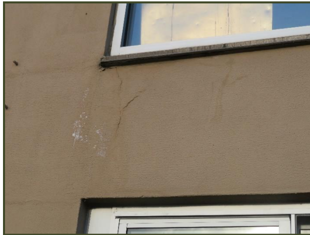
Photo No. 17 – Cracking and efflorescence at concrete framing
