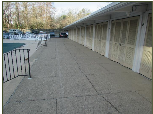
Photo No. 27 – Cracking in concrete pool deck perimeter walkway
