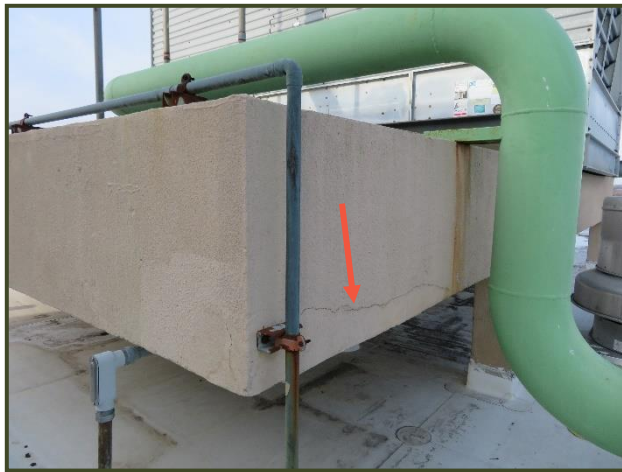
Photo No. 10 – Cracking on concrete equipment pad
