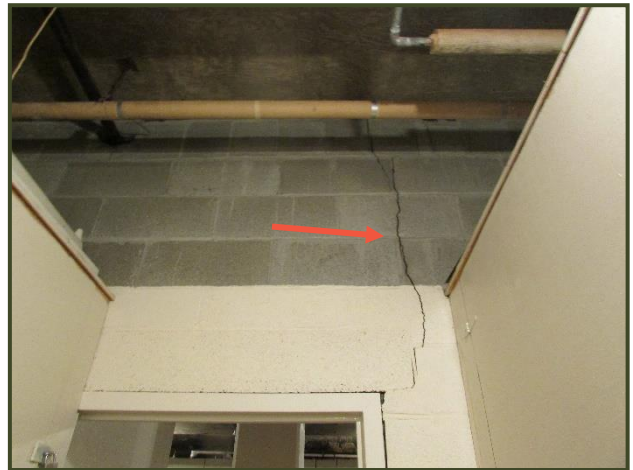
Photo No. 2 – Vertical cracking within CMU partition wall
