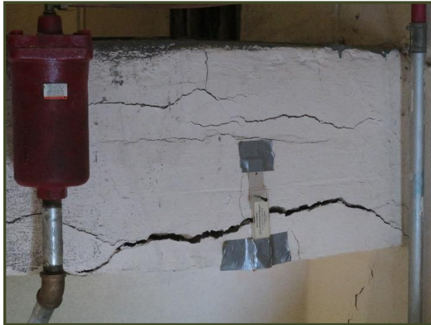
Photo No. 7 – Open cracking within concrete framing at top landing
