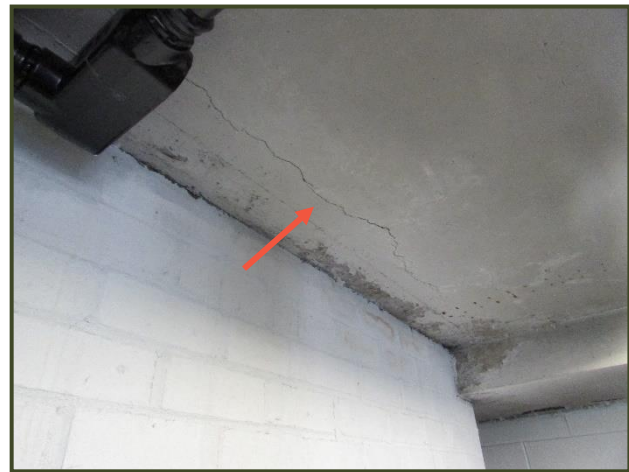
Photo No. 13 – Cracking at underside of penthouse roof
