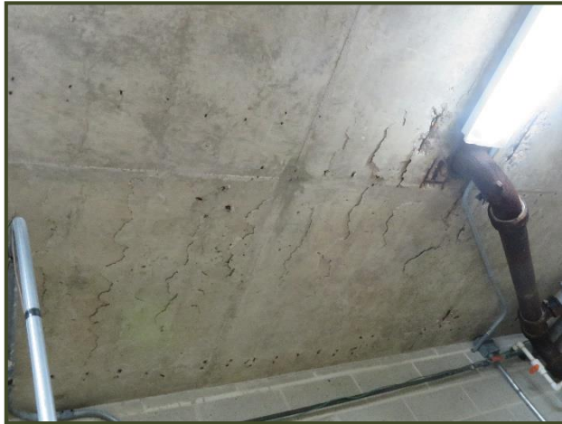
Photo No. 24 – Underside cracking and spalling at pool pump room ceiling
