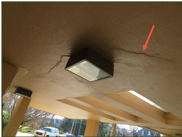
Photo No. 22 - Incipient spalling in underside of front entrance canopy
