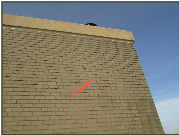
Photo No. 12 – Brick step cracking at exterior penthouse wall
