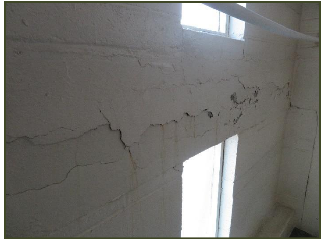
Photo No. 8 – Cracking, incipient spalling, and water staining at concrete framing
