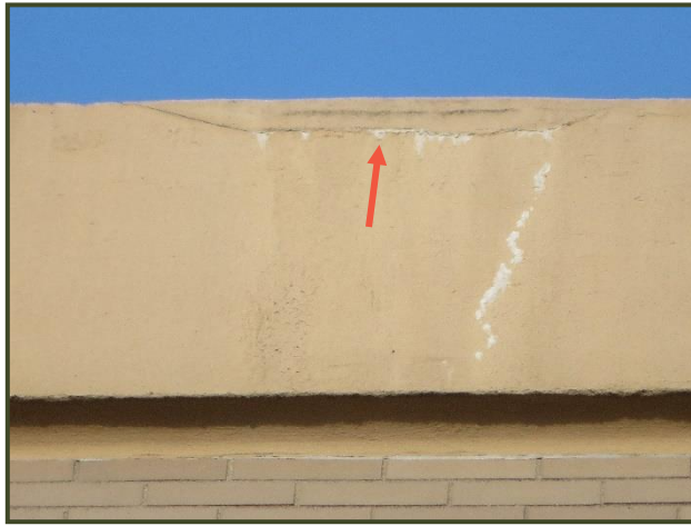
Photo No. 15 – Cracks and efflorescence on concrete roof framing
