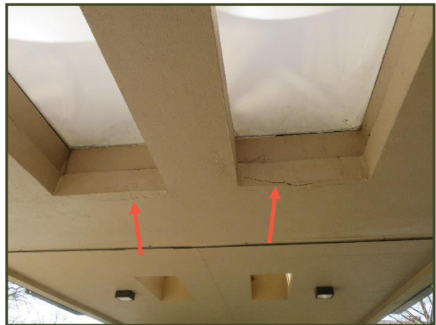
Photo No. 23 - Concrete cracking at underside of front entrance canopy
