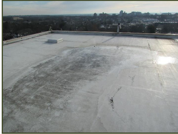
Photo No. 14 – Ponding on main roof surface
