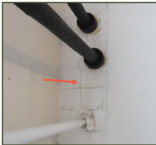
Photo No. 9 – Isolated cracking at CMU at pipe penetrations
