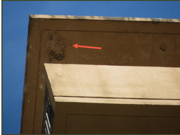
Photo No. 20 - Incipient spalling and peeling coating in underside of cantilever concrete balcony roof
