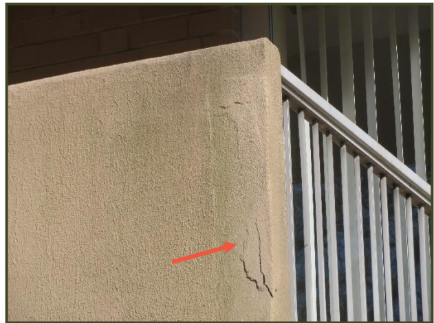
Photo No. 19 – Incipient spalling in concrete balcony wall
