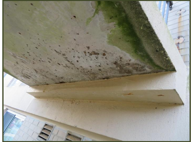
Photo No. 21 - Deterioration of underside of exterior concrete staircase
